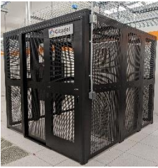
Servers locked in a cage as part of the Secure Research Infrastructure at Princeton University.
